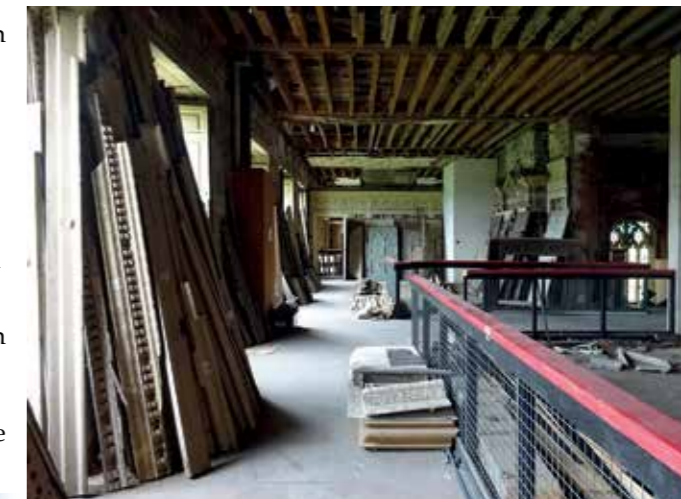
The historic rooms on part of the first floor have been dismantled with panelling and other components stored.
