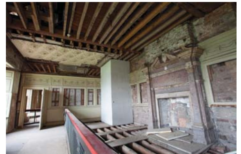
Ashton Court - Derelict First Floor
